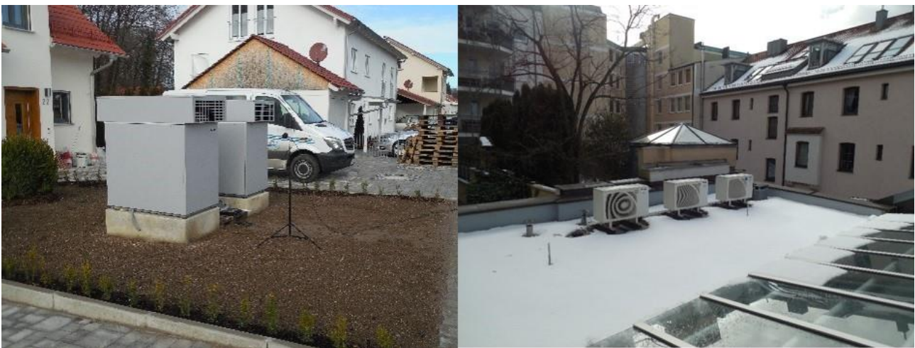
Figure 1 Typical stationary domestic service facilities in the residential environment (left: air heat pumps; right: air conditioning units)
