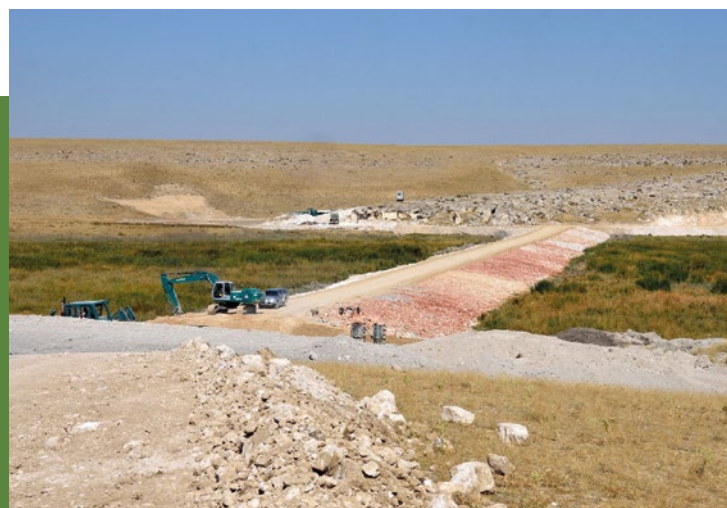
Construction of a dam to retain water in a valley mire in Turkey
