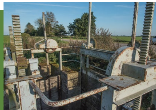
Old weir with visible need for repair in a fen
