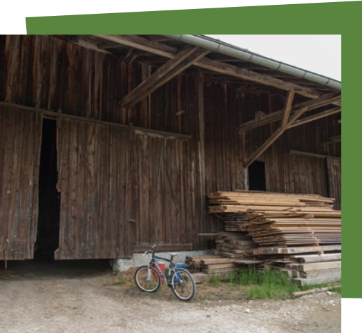
Clearly visible subsidence of the peat soil next to a barn on the peatlands
