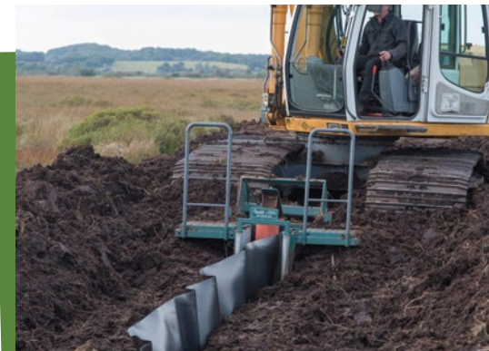
Rewetting of a raised bog; plastic sheet driven into a peat embankment to retain water
